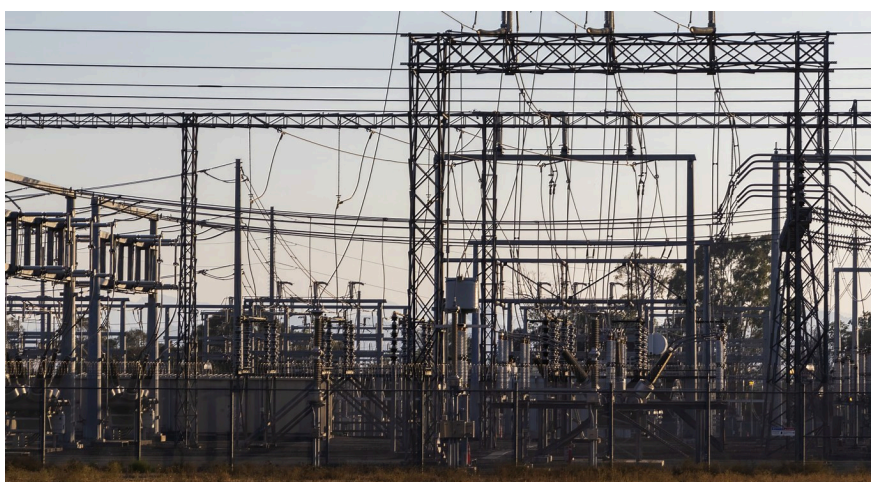
Campuses in the region increasingly connect at transmission voltages with substations on site. The engineer who owns that relationship with the utility comes from the power sector, not from information technology.
