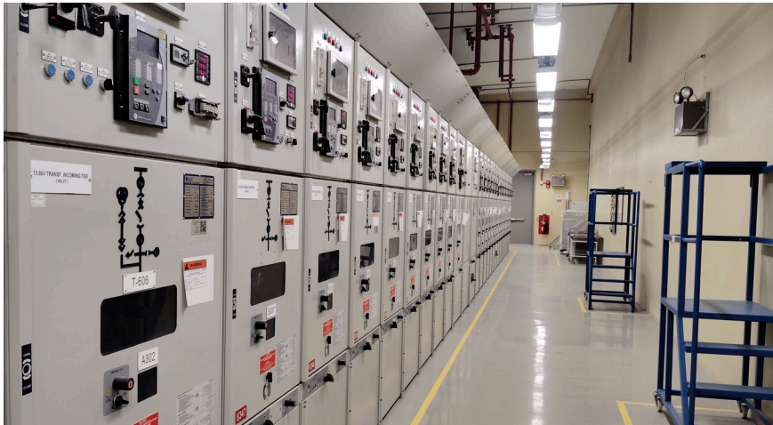
Switchgear panels labelled at 13.8 kilovolts. The roadmap described here would convert from that supply level straight to 800 volts direct current.
