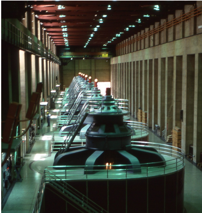
Rotating plant, electrical distribution, alarm management and the discipline of running shifts. A power station already teaches most of what the electrical side of a data centre will ask for.
